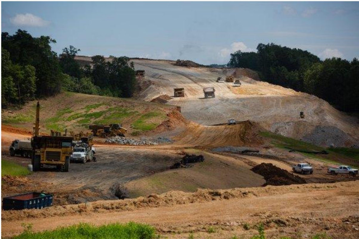
Construction on a road that will connect LakePoint's north and south campuses. The north campus is not yet built. Credit Kevin D. Liles for The New York Times
